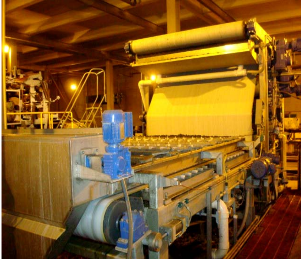
2 Meter Belt Filter Press – North Plant
