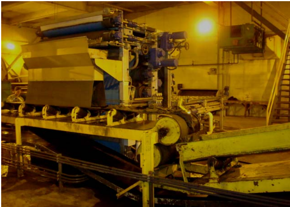
1.5 Meter Belt Filter Press – South Plant
