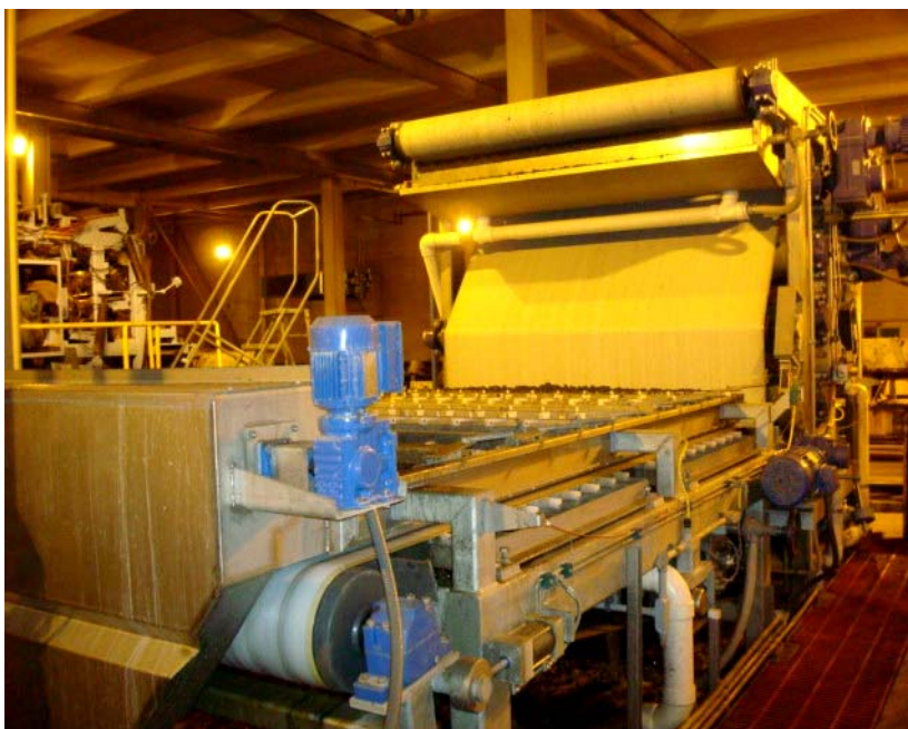
Two-Meter Belt Filter Press
