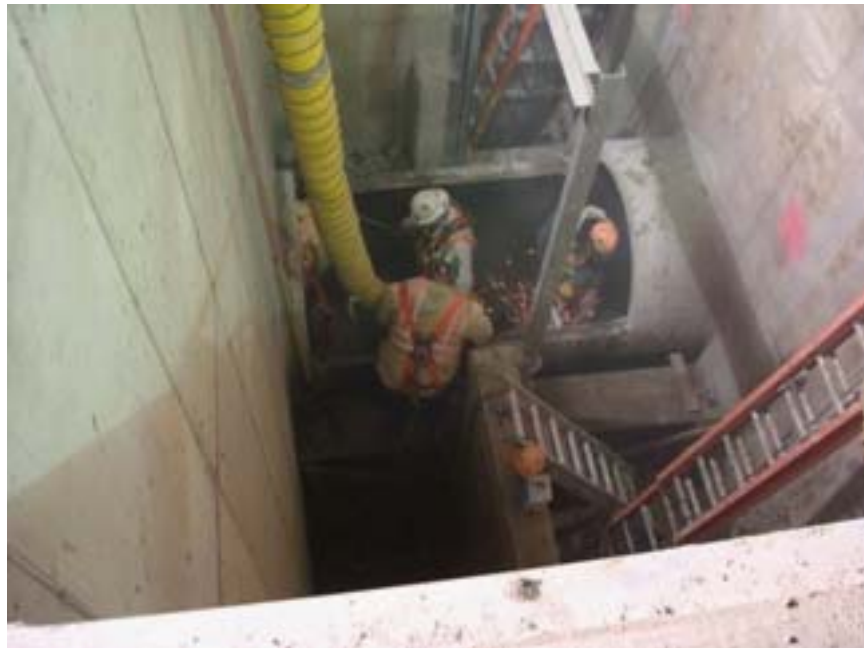
Diversion Chamber / District 60" Outfall Pipe
