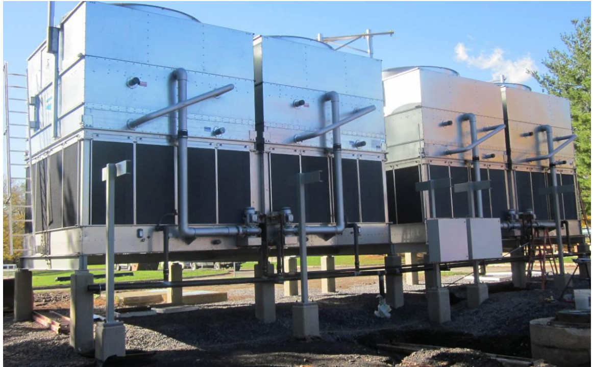
Installed Closed Circuit Coolers
