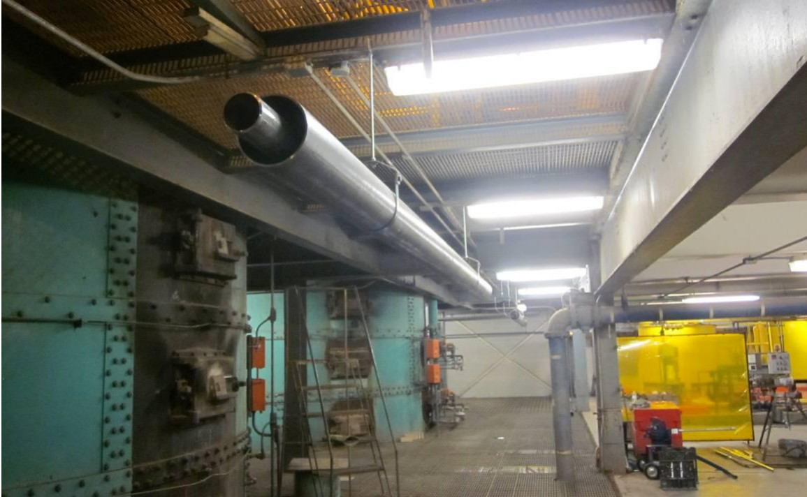
Hot Oil Piping
